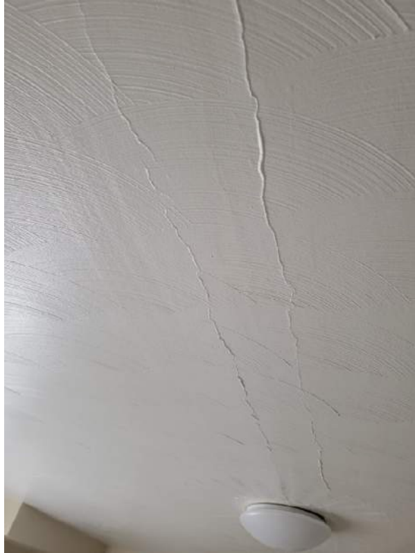
Typical ceiling crack in bedroom.
