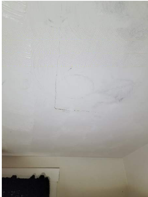
Typical ceiling crack in bedroom.
